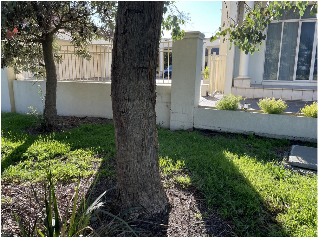
Image 19: Base of Tree 1758 (Red Box, front) and Tree 1759 (Coast Banksia, rear) in northeast lagoon park section adjacent to 15-17 Macquarie Circle showing cracking/damage to structure, possibly associated with tree roots. Trees recommended for removal.
