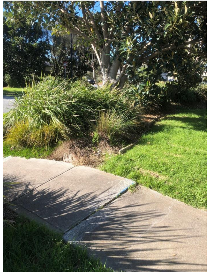
Image 21: Footpath lifting due to fig tree roots
