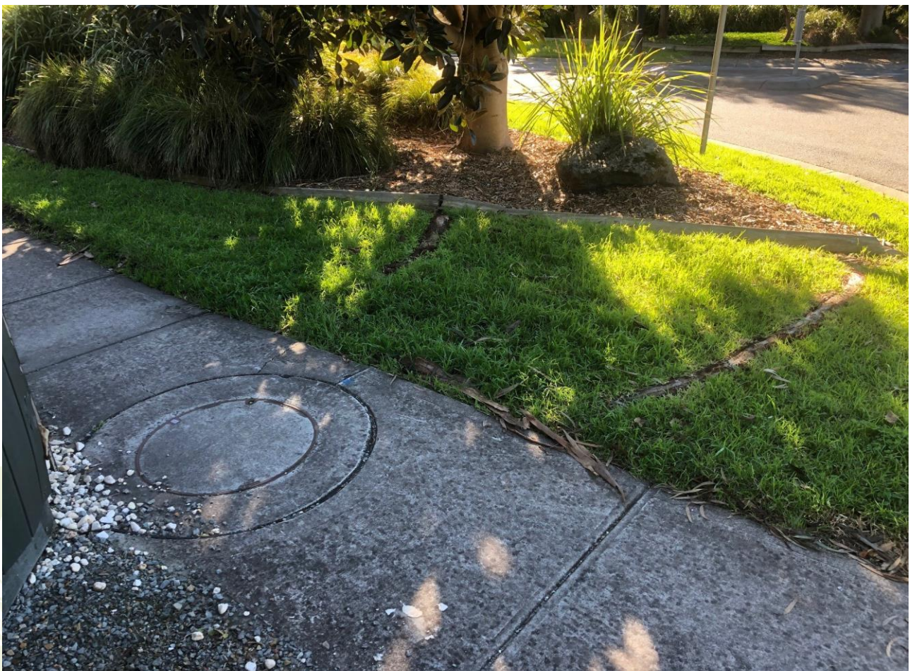
Image 22: Showing surface roots of fig tree and footpath panel lifting. Ongoing and major damage is increasingly likely as the fig trees mature. Trees have been recommended for removal.
