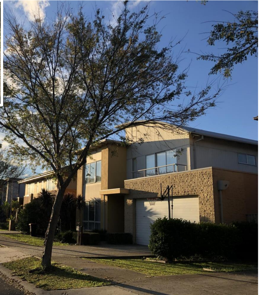
Image 7: Tree 338, Chinese Elm along Dresden Drive in overly small and narrow planting space causing footpath damage and likely to continue doing so. Recommended for removal. INSET: Closeup of footpath damage.
